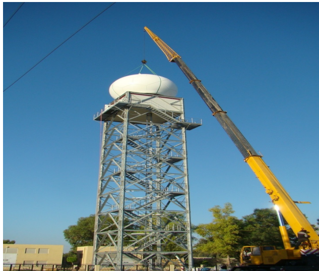
METEO. 500C weather Radar (Tripoli, 2008)
